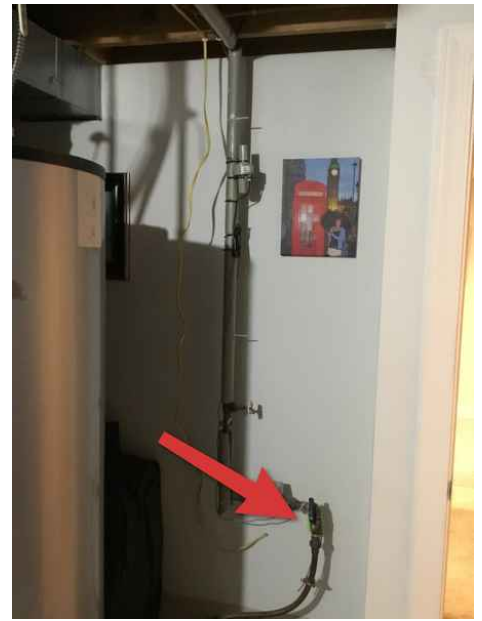
Water shutoff - Mechanical Room
