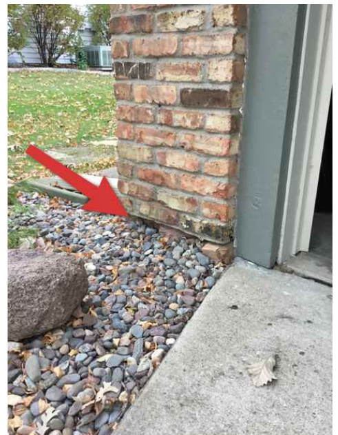
Missing brick - west of garage door
