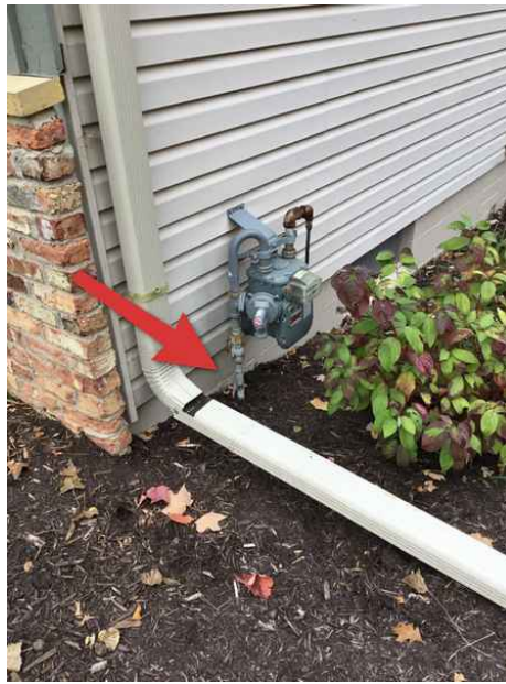
Gas Shutoff - East side of house
