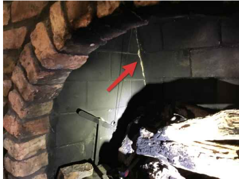
Crack in brick firebox
