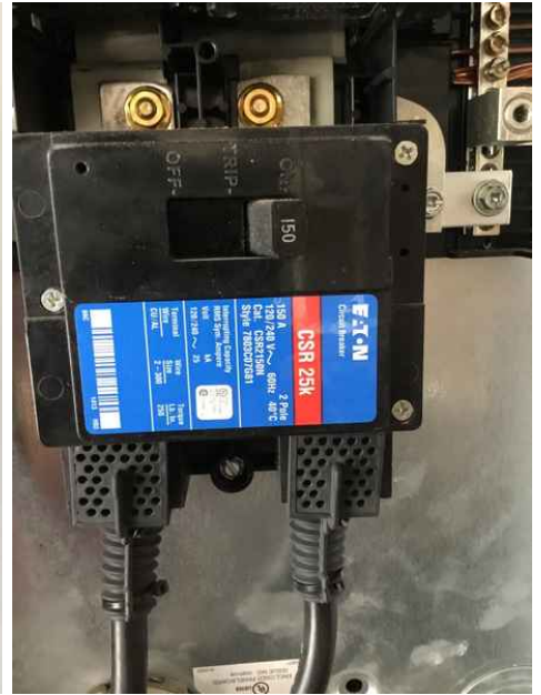
Main breaker (150 amps)
