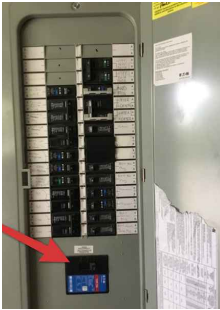
Main Service Panel
