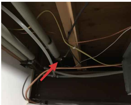
Shut off valve - Front hose bib
