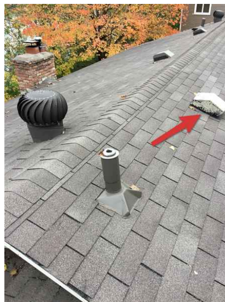
Exhaust vent for gas stove
