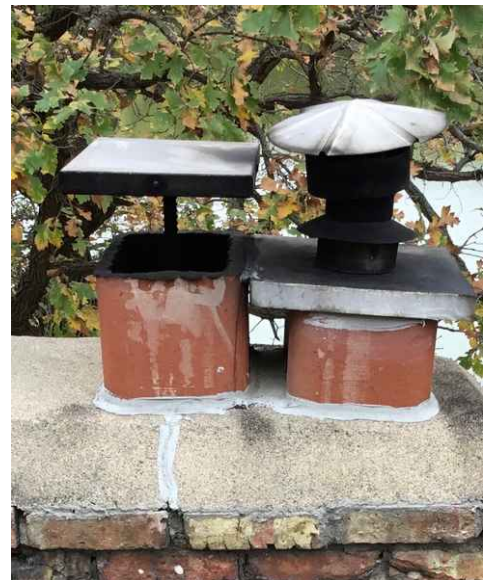
Installed cap limited accessibility to the flue.
